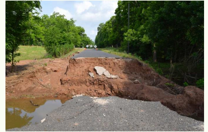
Floods - Texas, 2016 (FEMA News Photo)
